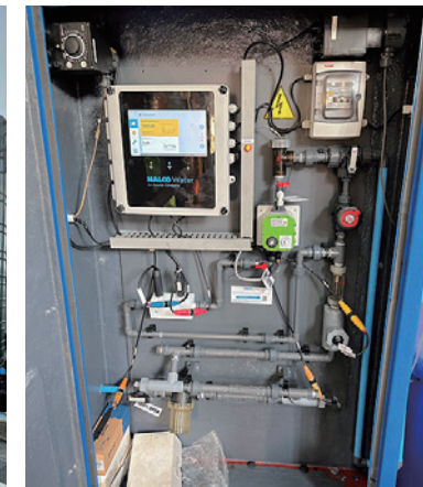
Water quality monitoring system
